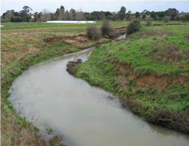
A lack of riparian vegetation and active erosion along the Hingaia channel
